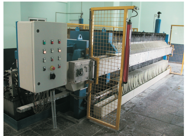
Sludge is being pressed in the chambers
