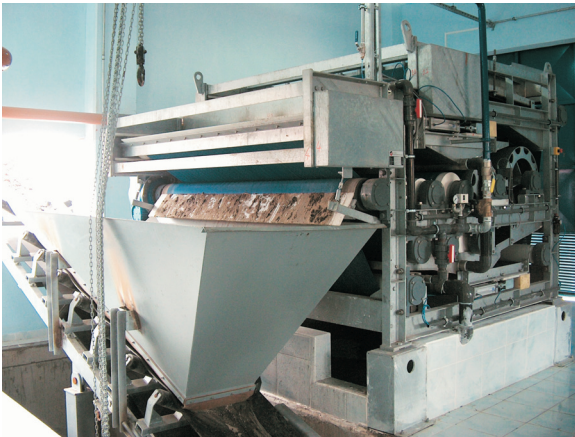
Sludge from Belt Filter Press is conveyed with belt conveyor
