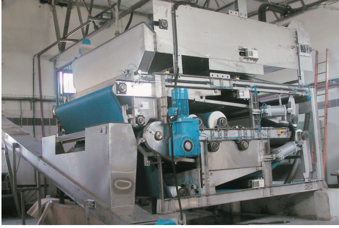
Gravity Belt Thickener and Belt Filter Press as Combined Unit
